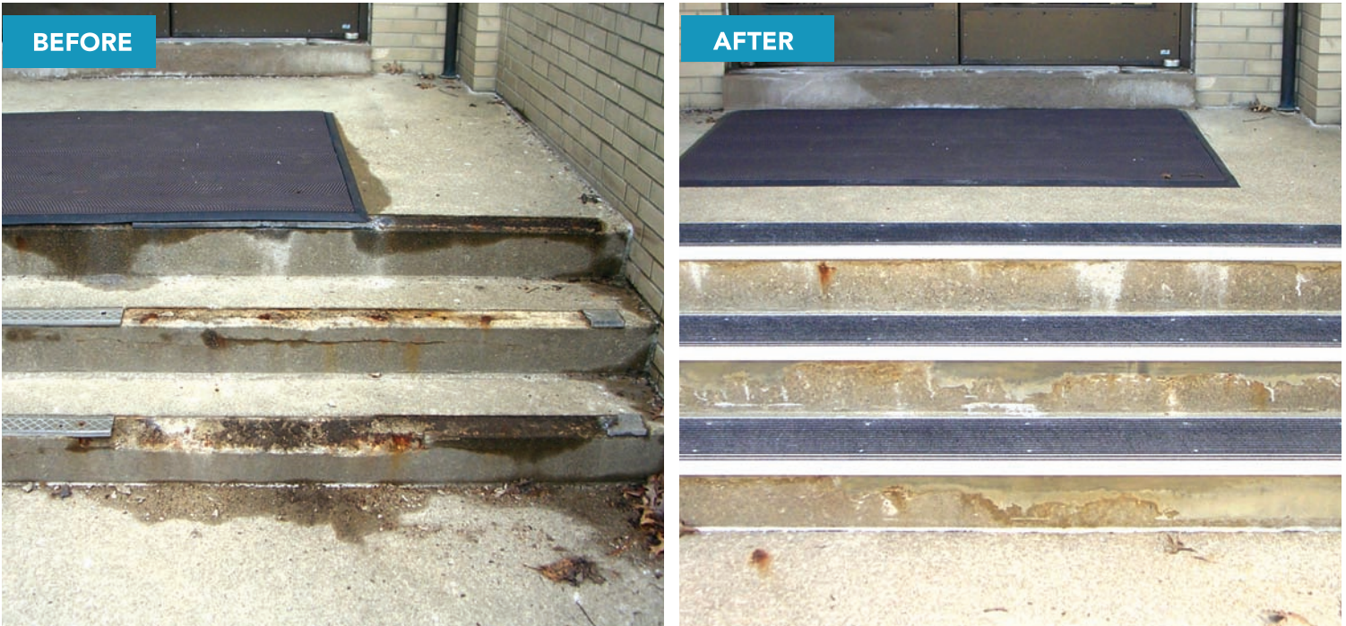
Left: Concrete stairs show their deteriorated condition before using renovation treads. Right: The stairs—with new renovation treads installed—have been restored to a safe condition.
